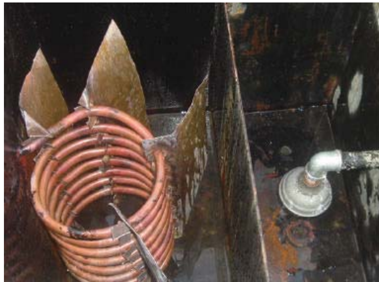
Fig. 5: Photo of desalination chamber
